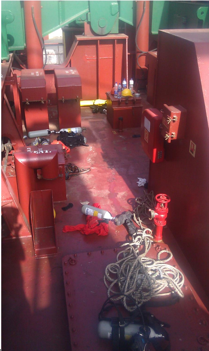
Sally Ann C – No.2 / 3 Cargo Hold Recess & Entrance to No.3 Cargo Hold Access Hatch
