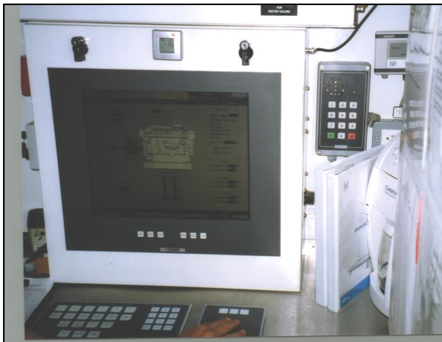
3. Engine Platform Management System on Main Engine Start Page
