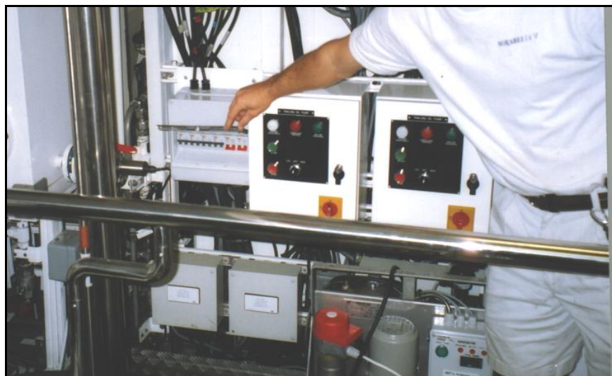
4. Main engine start electrical breakers
