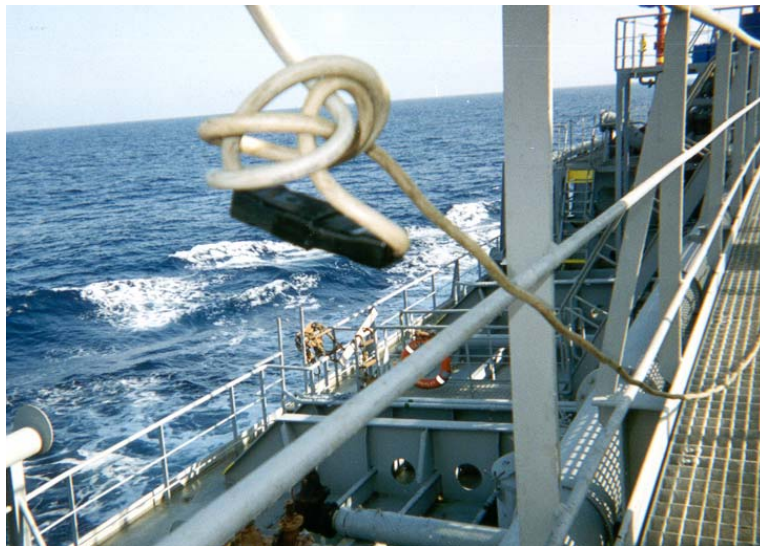
Photograph: The standard of electrical connection above tanks 9c and slop tanks.
